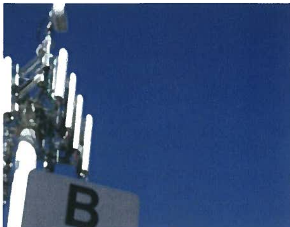
AT&T Sector 2 & AT&T Microwave
