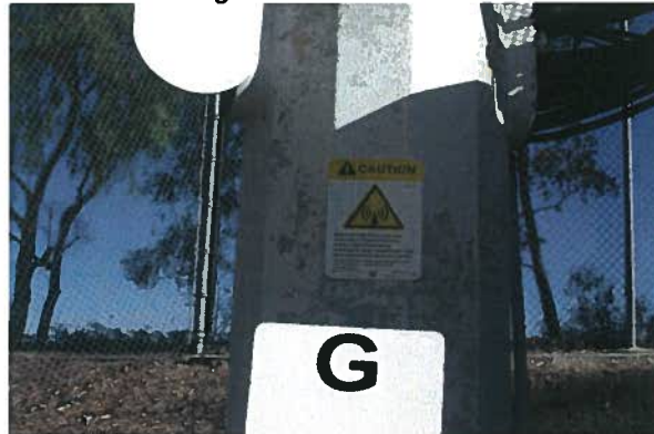
Sector3 Caution sign at the base of the monopole
