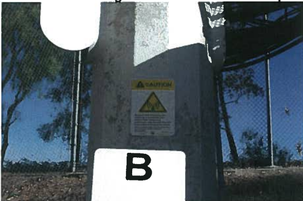
Sector2 Caution sign at the base of the monopole
