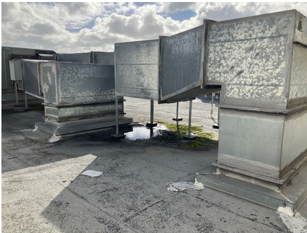
Standing water on the roof
