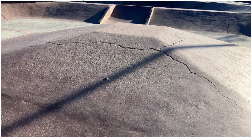
Example of Cracks in Skate Park Bowl
