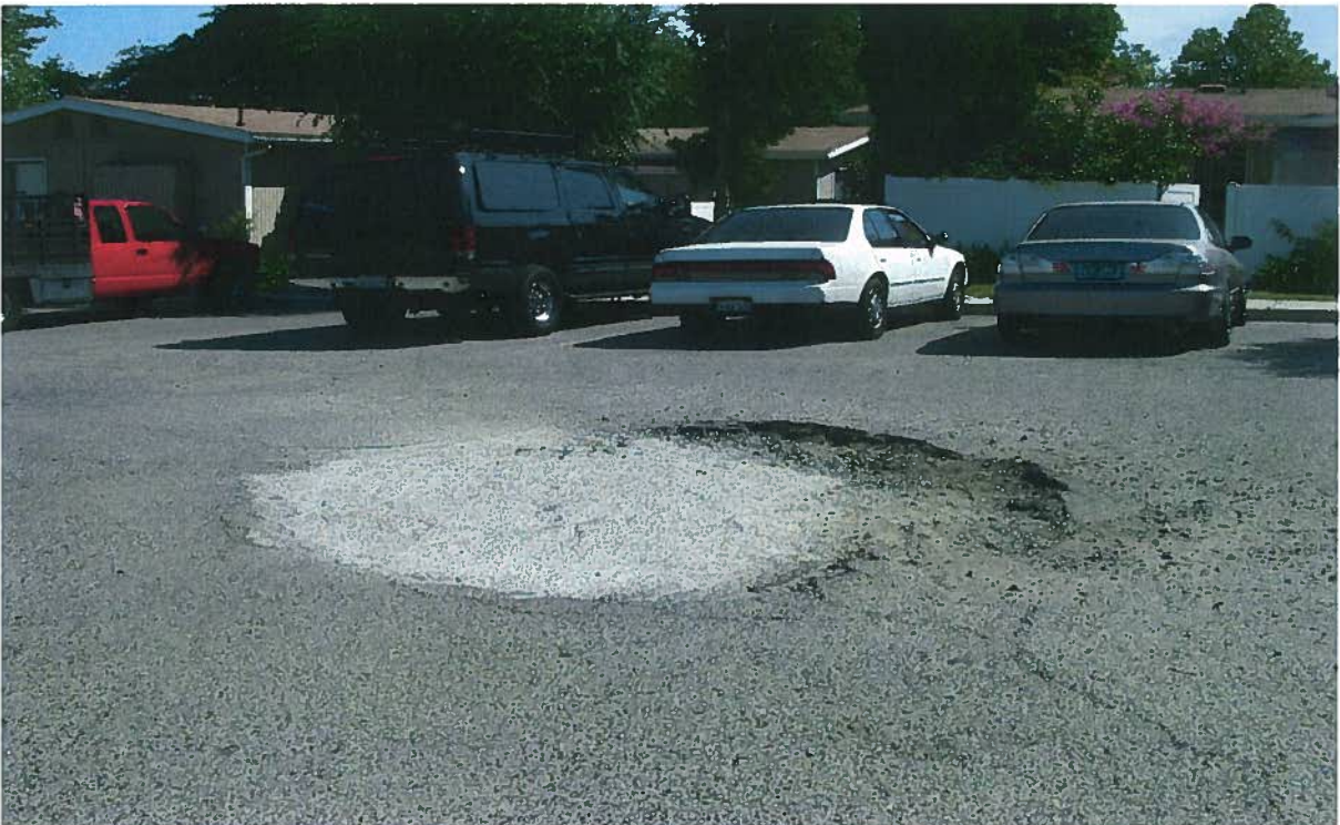
Parking Lot Pot Holes
