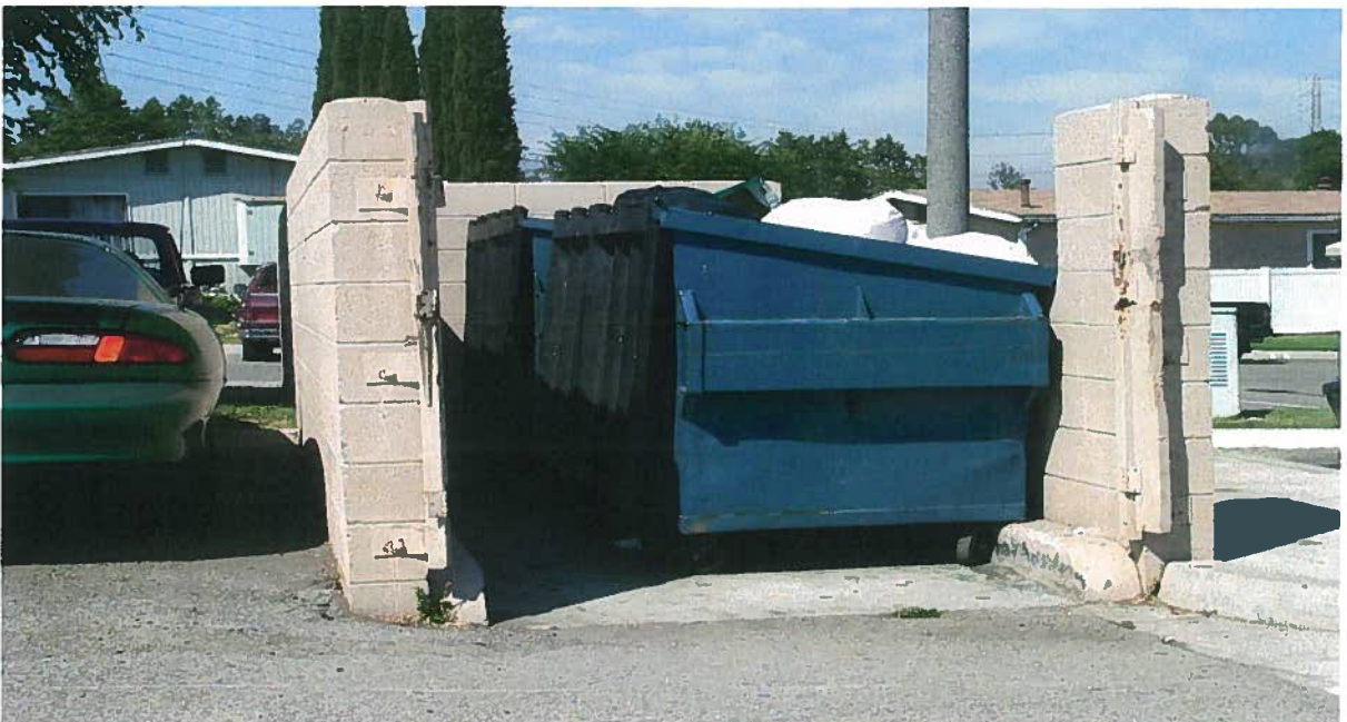
Dilapidated Trash Enclosures
