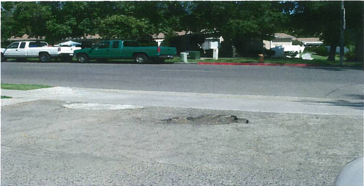
Parking Lot Pot Holes
