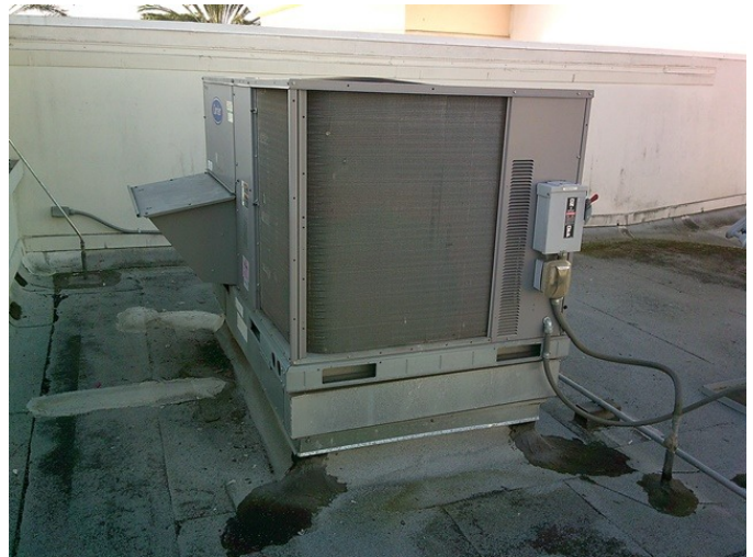
Package Unit on Roof
