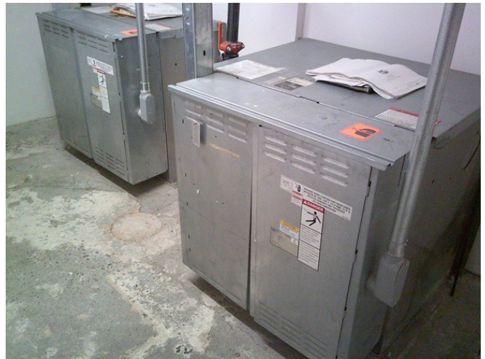
Elevator Hydraulic Pumps
