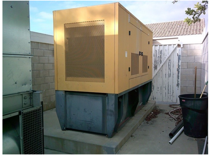
Emergency Diesel Generator
