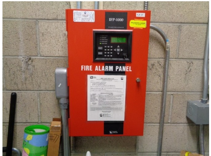
Fire Control Panel
