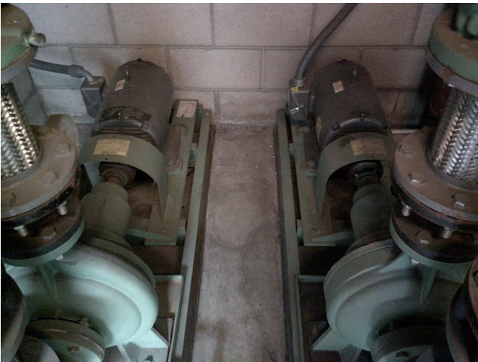
Pumps (Cooling Tower)
