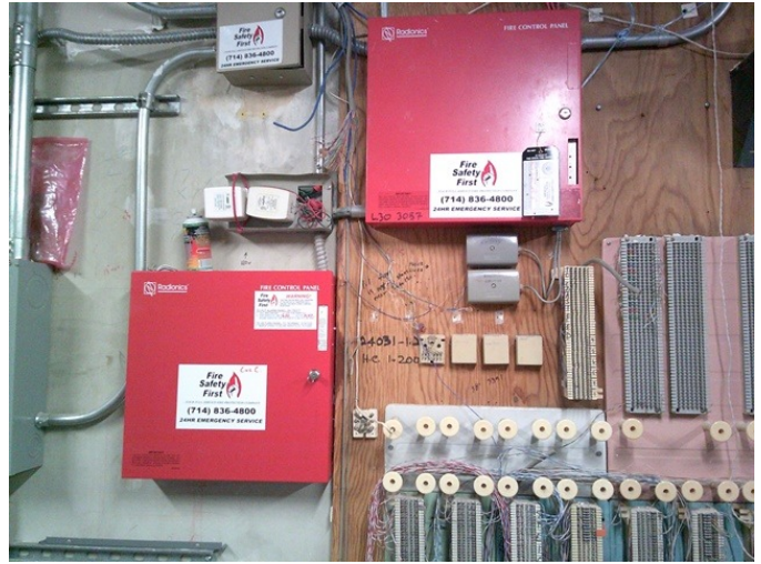
Fire Control Panel
