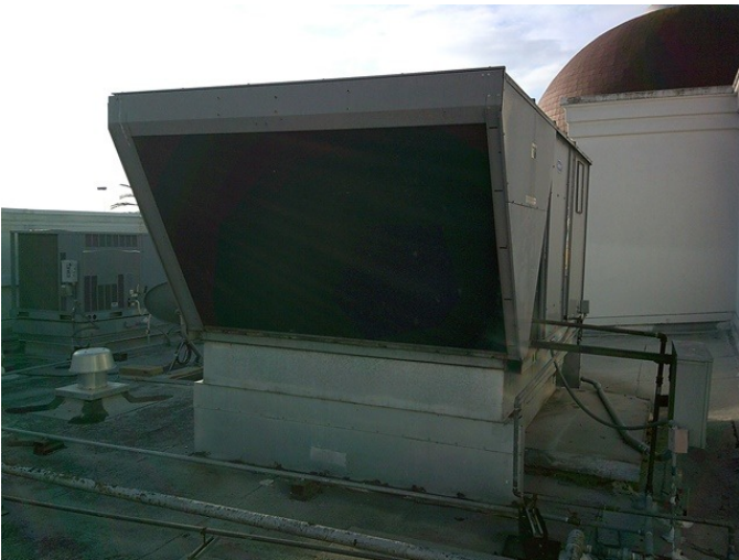
Package Unit on Roof
