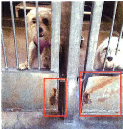
Examples of substantial rust and other damage on front kennel doors.
